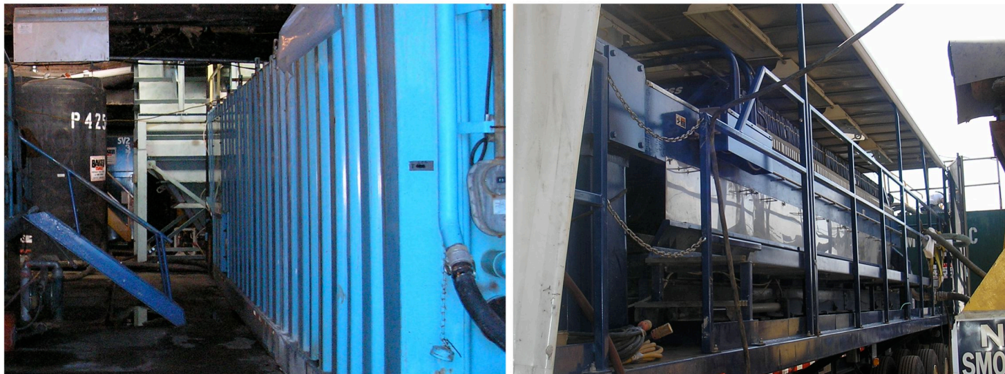
Wastewater Treatment Equipment (clockwise from top: Centrifuge Two and Conveyor, Filter Press, Lime Addition Tank)
