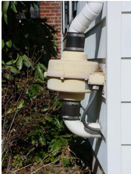
A subsurface depressurization system fan on the outside of a building.
