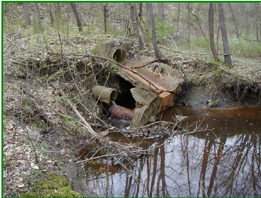
These badly eroded outfalls receive stormwater from the Flying "W" Airport.
