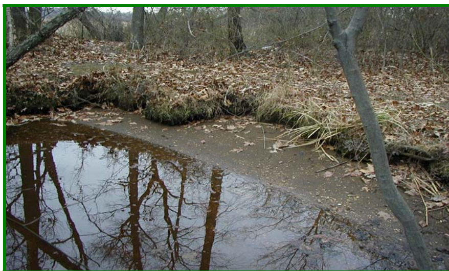
Tidal effects and the current have contributed to the erosion occurring along shoreline.
