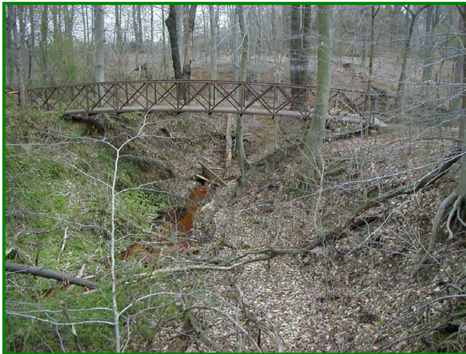
The stability of this footbridge has been compromised as the underlying ravine worsens due to the ongoing erosion.
