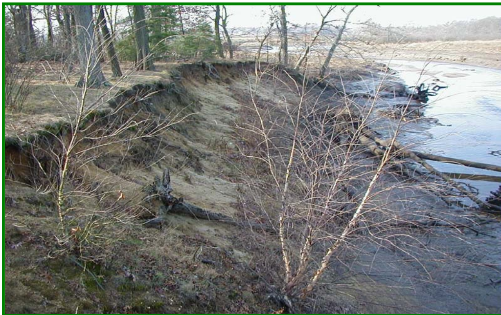
Sandy soils, poor vegetation, and upper bank failure has resulted in a significant eroded area at this location.
