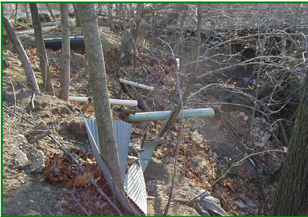
A multitude of protruding pipes and the failing condition of the slope can be easily seen in this photo.
