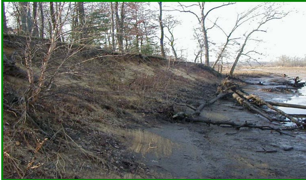
Many trees litter the shoreline at this site.
