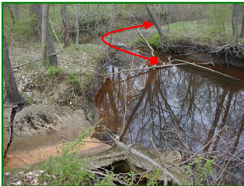
The eroded nature of the feeder stream can be easily seen in this photo.
