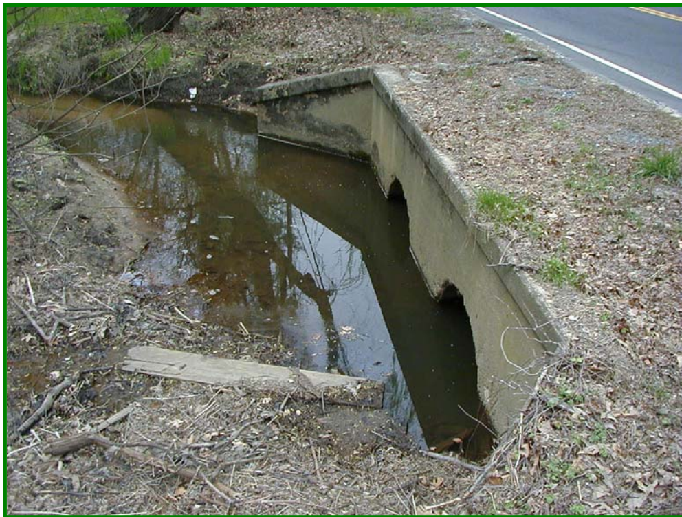
This culvert is blocked with sediment and other debris creating a flooding problem during times of heavy rainfall.
