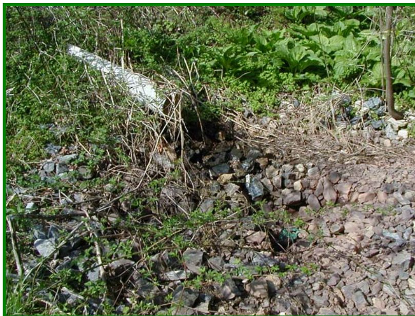
This outlet discharges to an inadequately stabilized area at the top of a slope.
