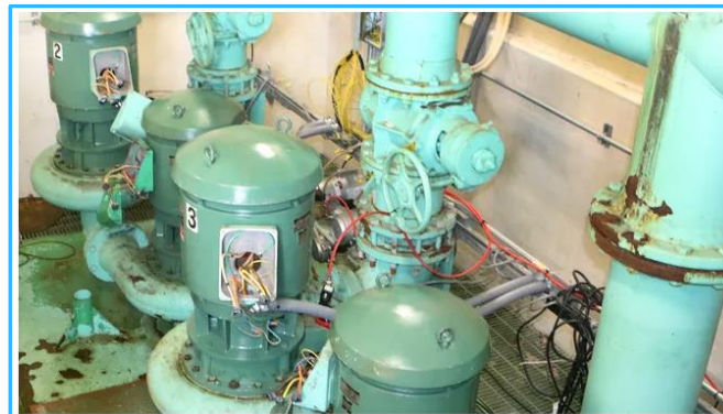
All six pumps housed in Pump Station #7 in Dover were submerged during a sewage leak and rendered inoperable. Jerry Smith/The News Journal
