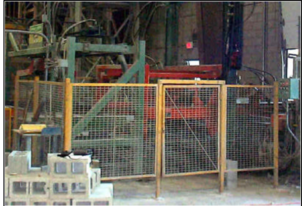
Fenced-in machine guard around machines
