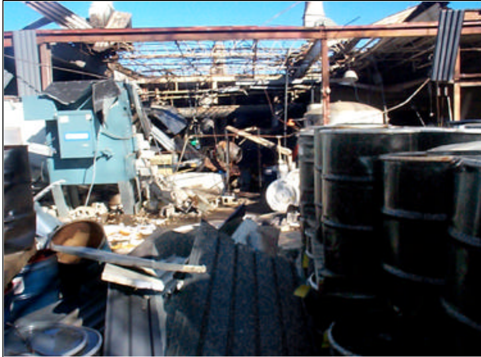
Photo 5 Acid Room Shortly After the Explosion
