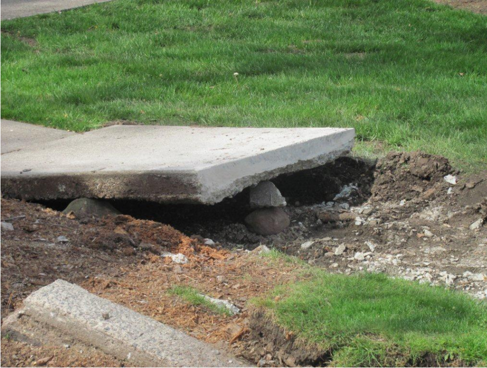
FIGURE 2: Sidewalk slab propped-up by stones.
