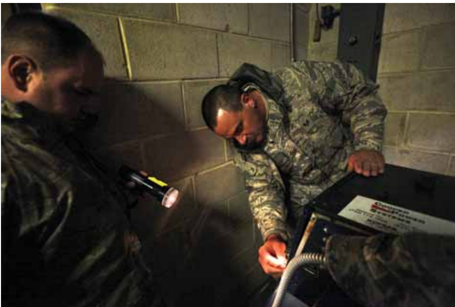
Photo below: Staff Sgt. Robert Jentsch, left, shines a flashlight onto the control panel of a gas-fired generator for Staff Sgt. Carl Hilpl, both with 108th Wing, as Hilpl prepares to start the system so the shelter at Veterans Memorial Middle School in Brick, N.J. will have power Nov. 7, 2012. Since Hilpl and his team of electricians came on duty, they have been hooking up generators and making sure they were compatible with existing electrical systems. Hilpl was also responsible for bringing oxygen tanks to a woman with cancer, every 12 hours for several days. (Air National Guard photo by Master Sgt. Mark C. Olsen/Released)
