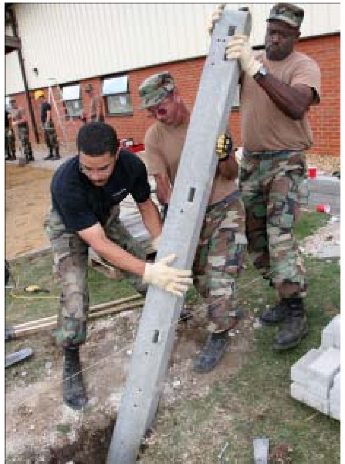
Left to right: Senior Airman Stephen Lee directs while Master Sergeants' Paul Nieczpiel and Raymond Gordon lower a fence post at the new gazebo.
