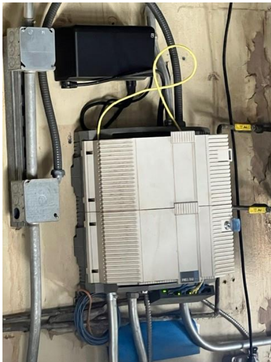
Existing BMS to be Upgrade
