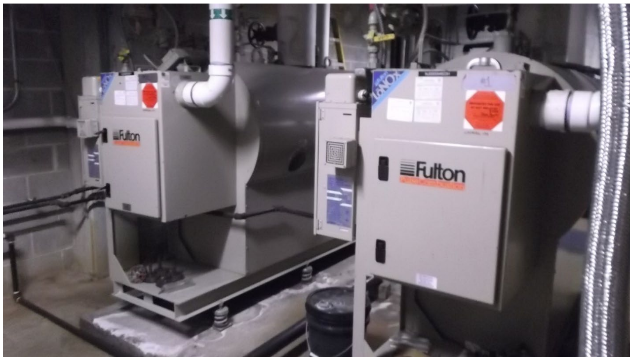
Fulton Boilers located in basement mechanical room.
