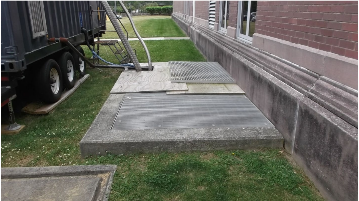
Outside view of air vent. Temporary rented boiler on the left.
