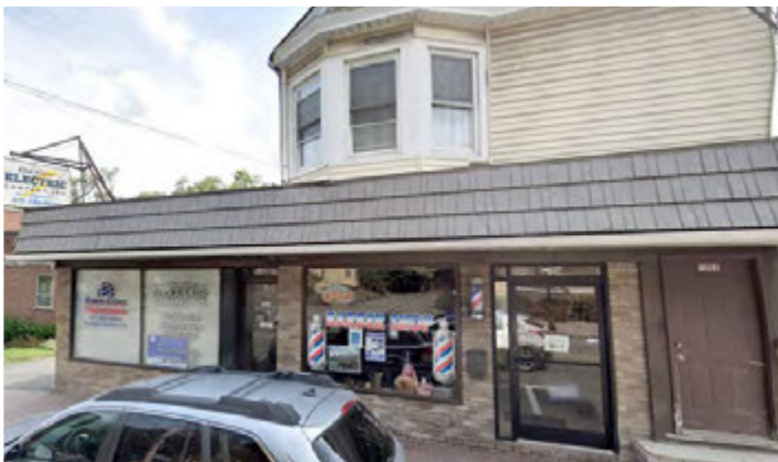
Figure 11: Building facade and storefront showing the need for maintenance.
