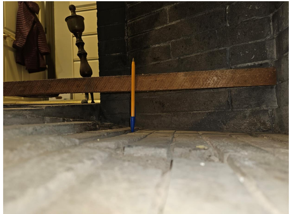
Inside fireplace showing slumping
