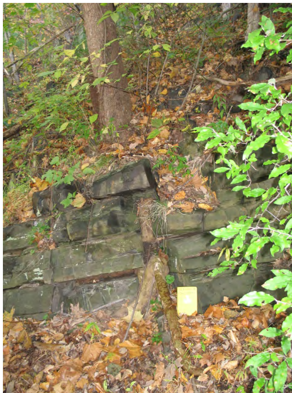
Photo 12 - Example of Root Wedging (Toe of Slope, Area D, Looking Northeast)
