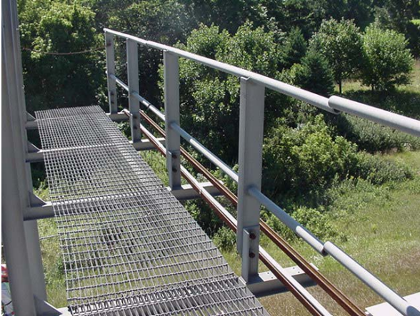
Figure 6. Catwalk with Safety Rails in Upright Position (Source: WSDOT, Structure Inspection Manual Part 4)
