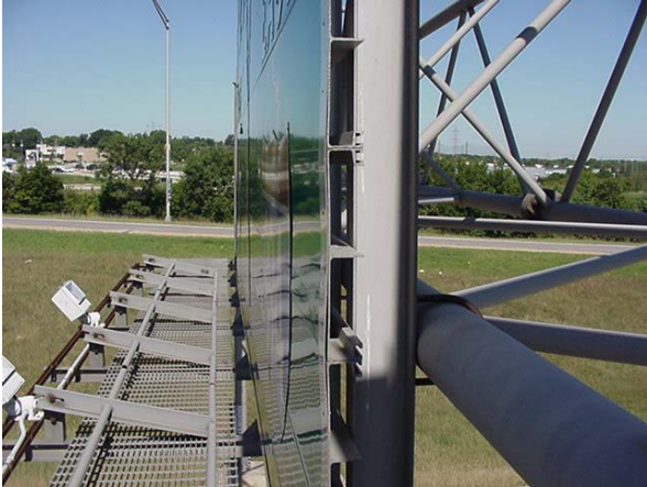
Figure 5. Catwalk with Safety Rails in Collapsed Position (Source: WSDOT, Structure Inspection Manual Part 4)
