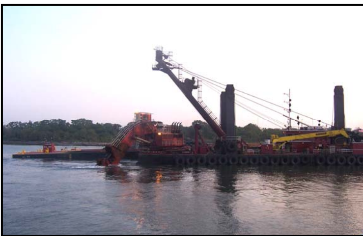
The Dredge New York, owned and operated by Great Lakes Dredge and Docking Company works on the Arthur Kill deepening project.
