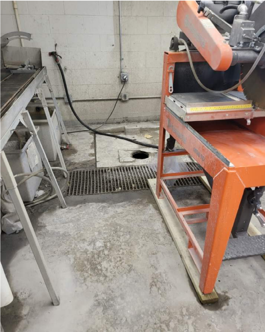
Existing Preparation and Batching Equipment. Note Washout Drain
