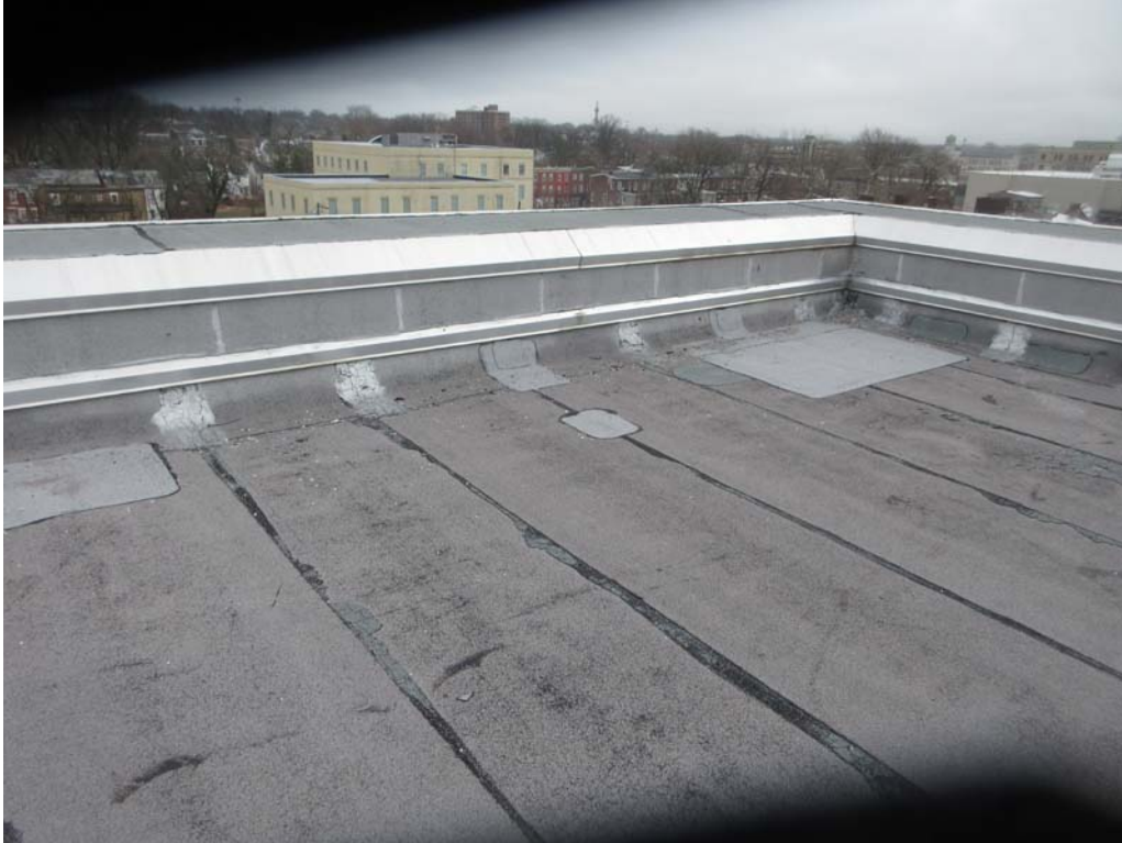
3. Roof Area B: Another section of Area B with more repairs.
