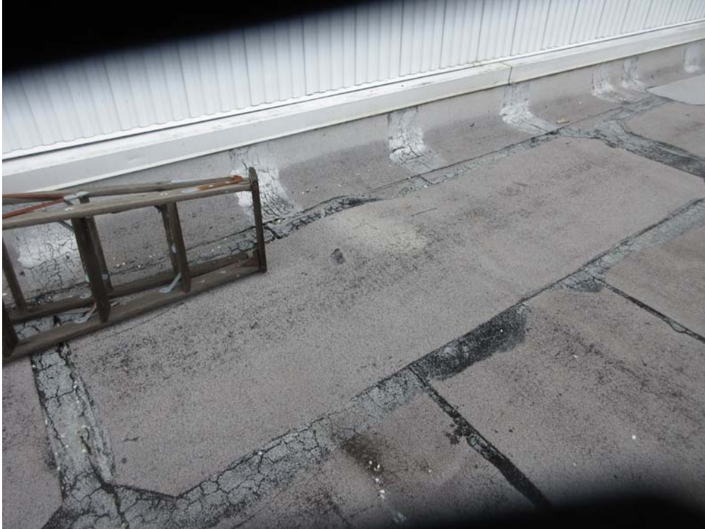
13. Roof Area B: View showing a blister at the inside wall on Area B along with previous repair attempts.
