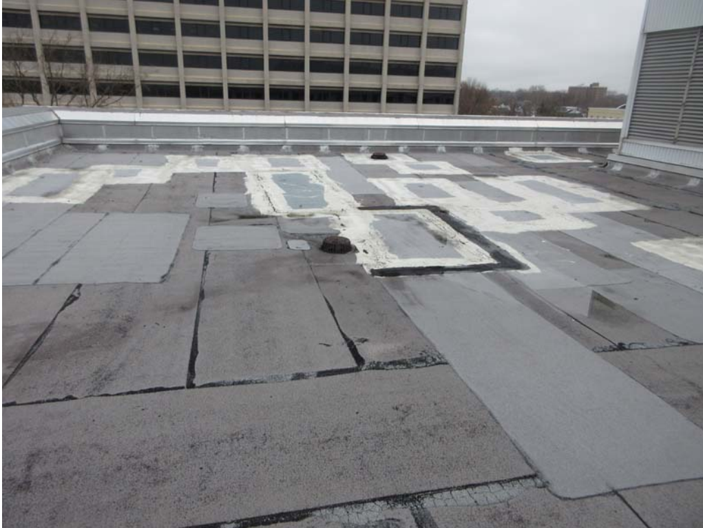
9. Roof Area B: Another overall view of numerous repairs made within the field and perimeter.
