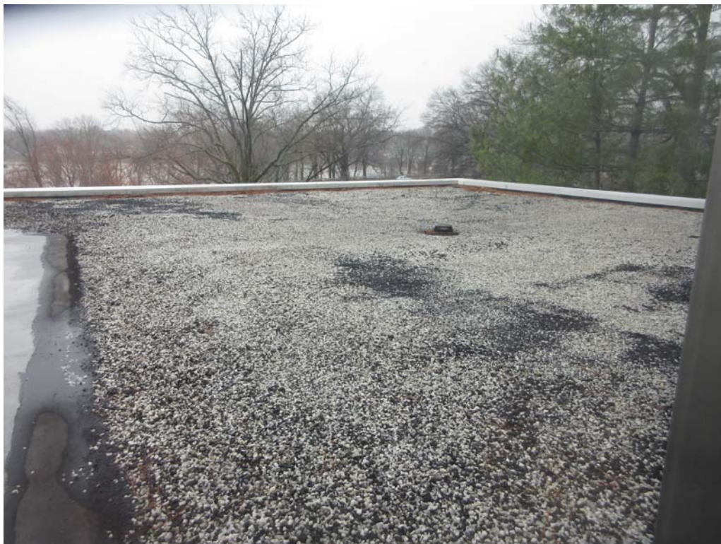
2. Roof Area C: Another overall view adjacent to the repaired area seen in photograph #1 above. The roof system on Area C is degraded and should be replaced as soon as funding is available.
