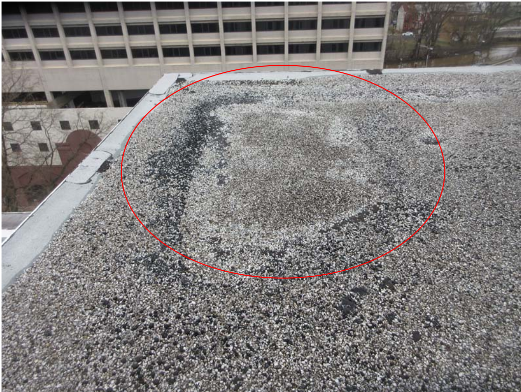
8. Roof Area A: Another section of Roof Area A whereby repairs were made with new materials.
