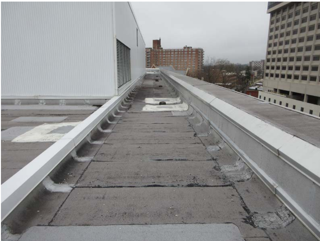
6. Roof Area B: Partial view of Area B showing more repairs and numerous membrane blisters.
