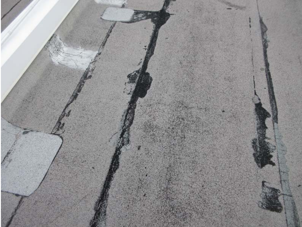
5. Roof Area B: Close-up view of an elevated membrane blister on Area B.
