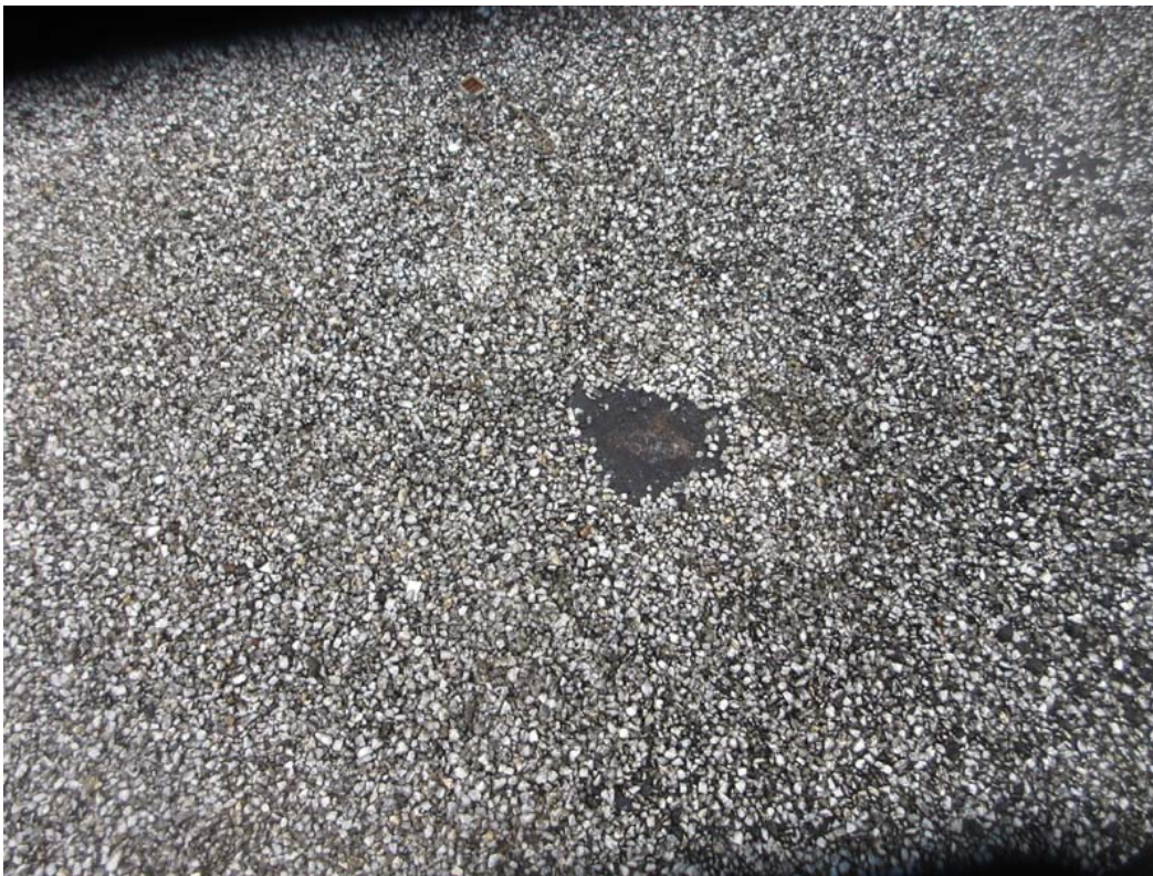
6. Roof Area A: Another close-up of an elevated blister in the field of the roof. The protective aggregate surfacing has eroded away.
