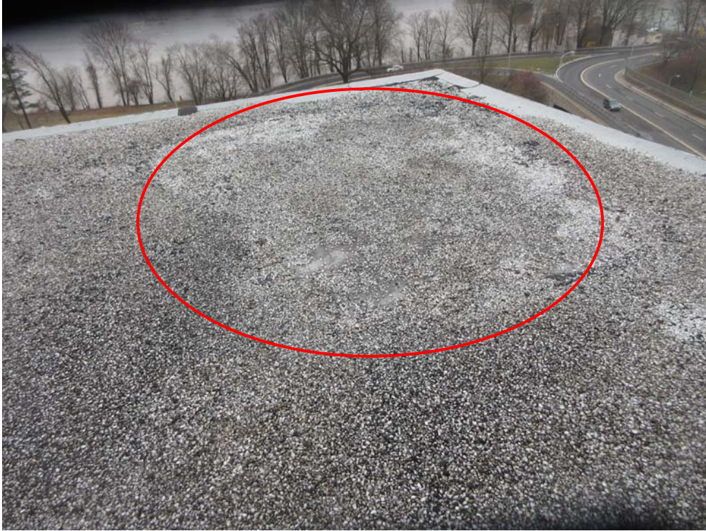
7. Roof Area A: View showing a large section of Area A where repairs have been performed to stop leaks.
