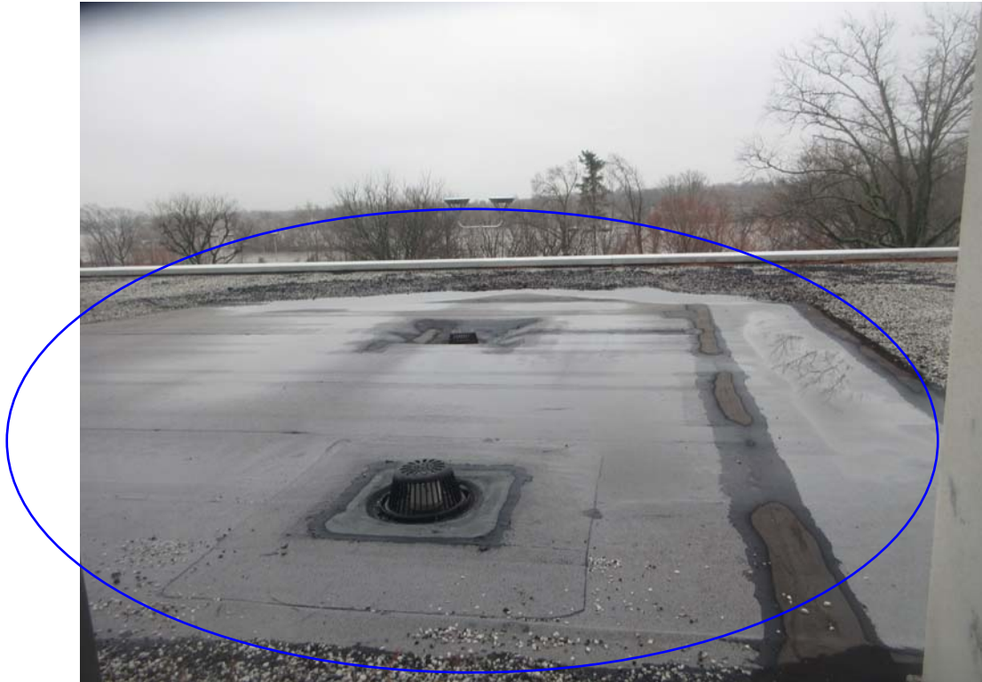
1. Roof Area C: Partial overall view of Area C showing a recent large repair made in the field.
