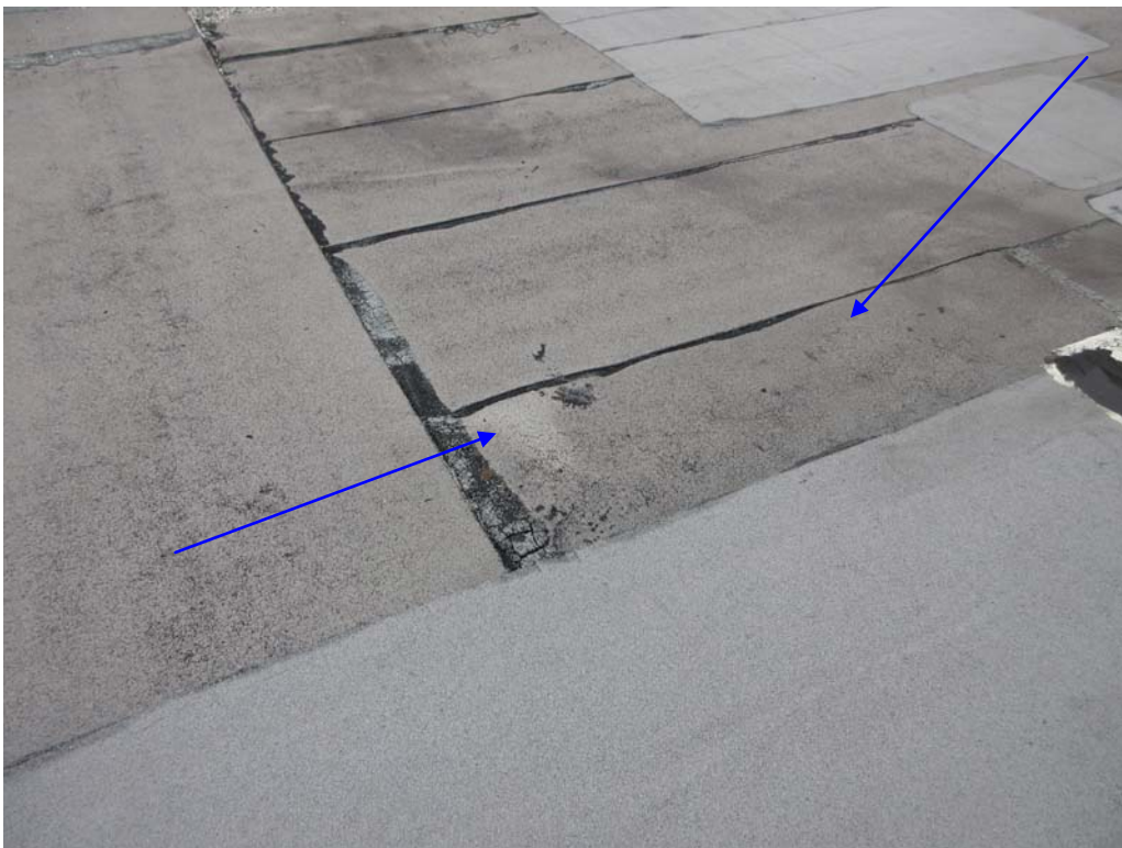
10. Roof Area B: Close-up view of membrane blistering.
