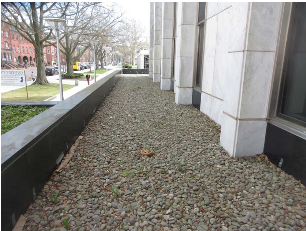
1. Roof Area D: Partial overall view of the ballasted EPDM roof system on Roof Area D.
