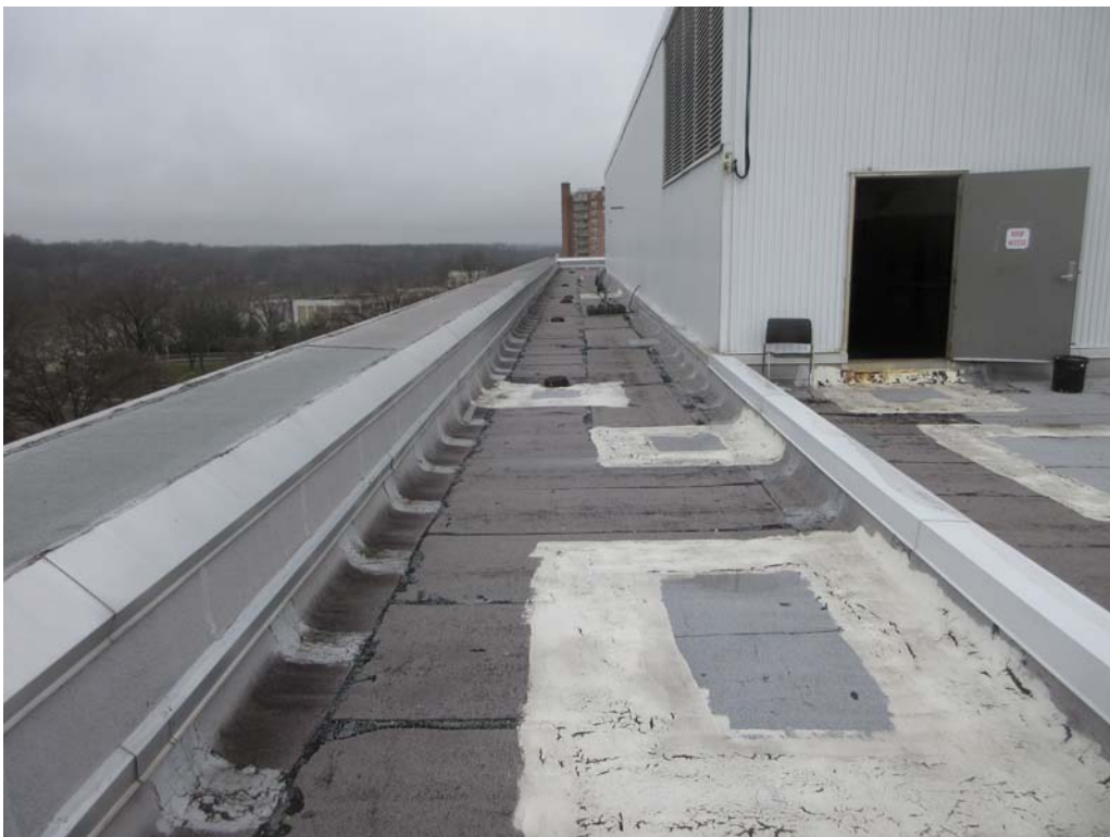
4. Roof Area B: Alternate view of Area B showing more repairs. Note the white material utilized for repairs which indicates that it was performed more recently than the other repairs.
