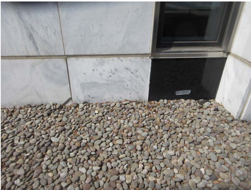
5. Roof Area D: Close-up taken at the base of the building wall panel showing the ballast above the bottom of the panel.
