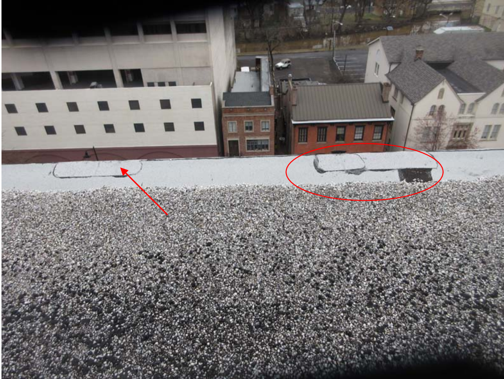
5. Roof Area A: Previous repairs were noted at the perimeter.
