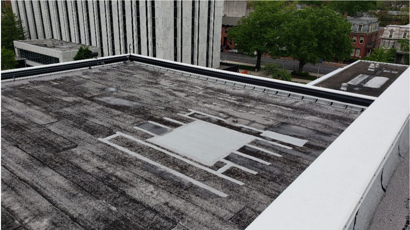
Main Roof West Side. Previous Patch
