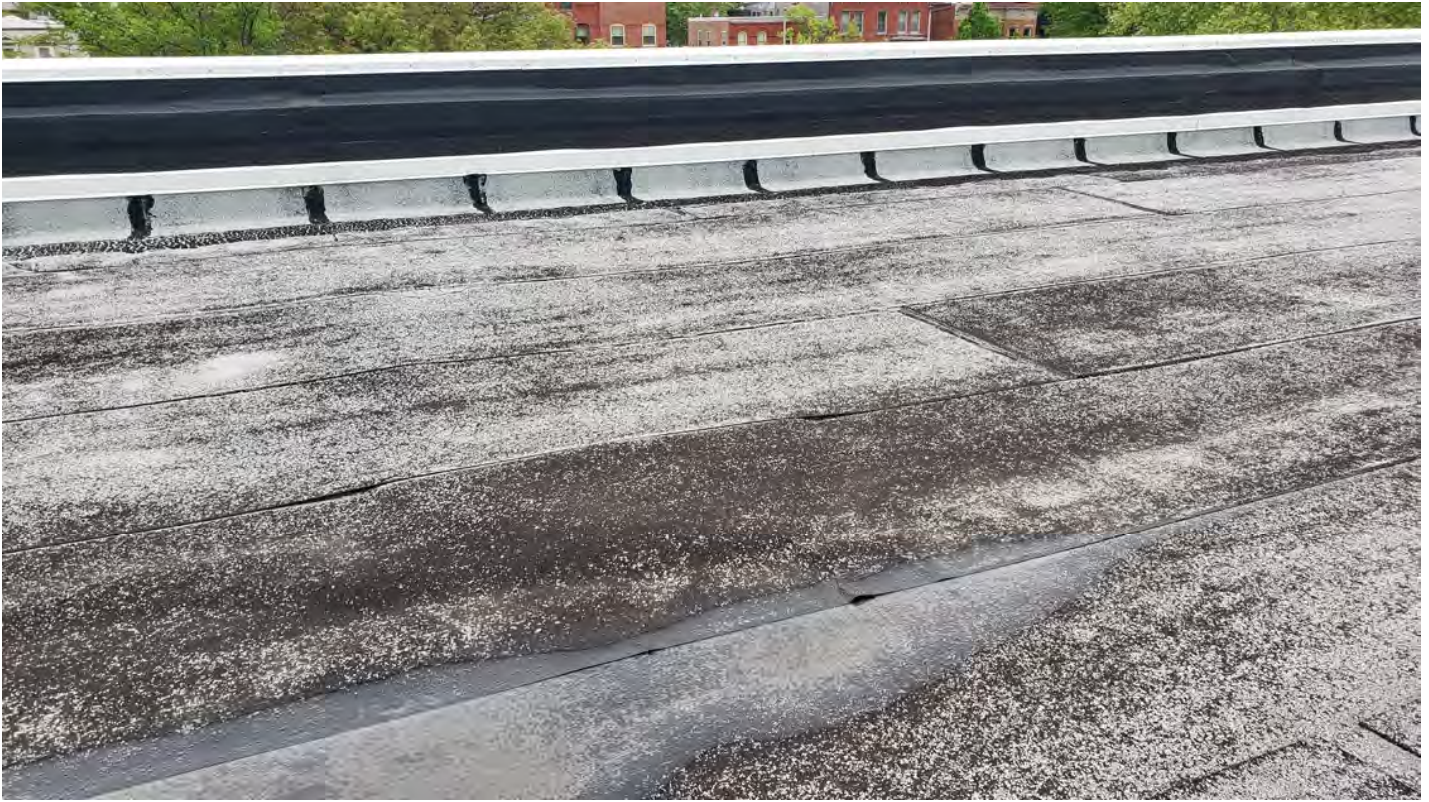
Standing Water, Fishmouthed Ply Edge, Loss of Surface, and Bubble
