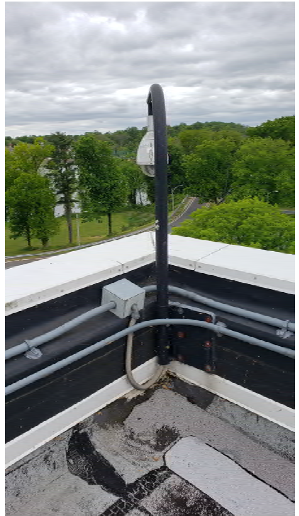
Camera at Main Roof Parapet
