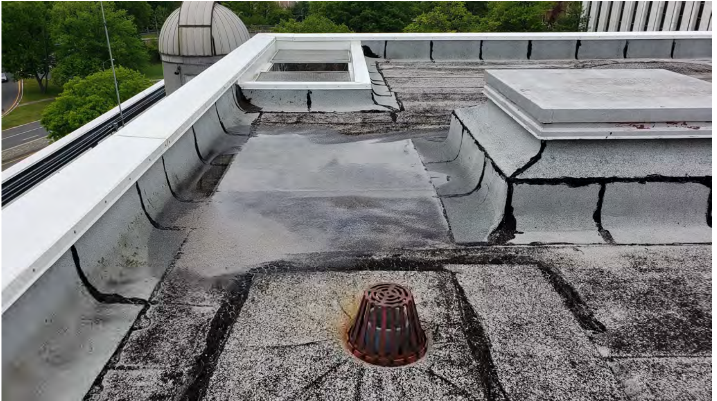
Standing Water and Overflow Roof Drain at Penthouse Roof
