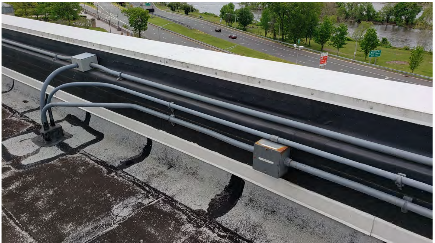
Conduits Rise From Run Within Roof Insulation Through Pitch Pocket and Run Along Parapet
