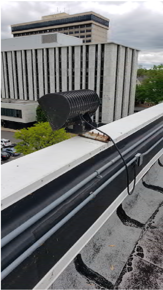
Light Fixture and Conduits at Main Roof Parapet
