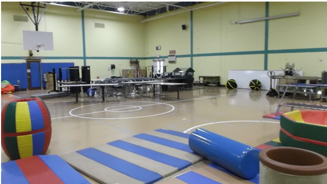
Gymnasium Rubber Floor to be replaced
