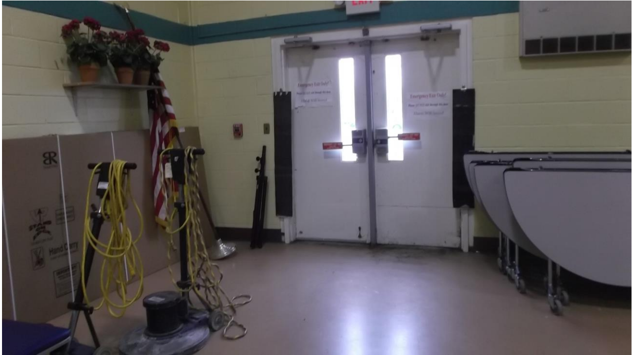
Gymnasium Rubber Floor along Exterior Double Doors to be replaced.
