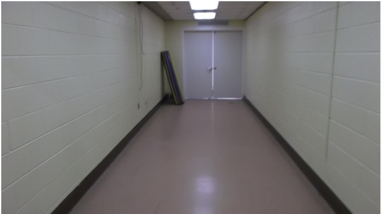
Connecting Hallway between Gymnasium and Main School Corridor Rubber Flooring in this Hallway to be replaced.
