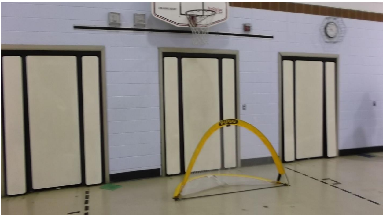
Gymnasium Worn Flooring under Basketball Hoop
