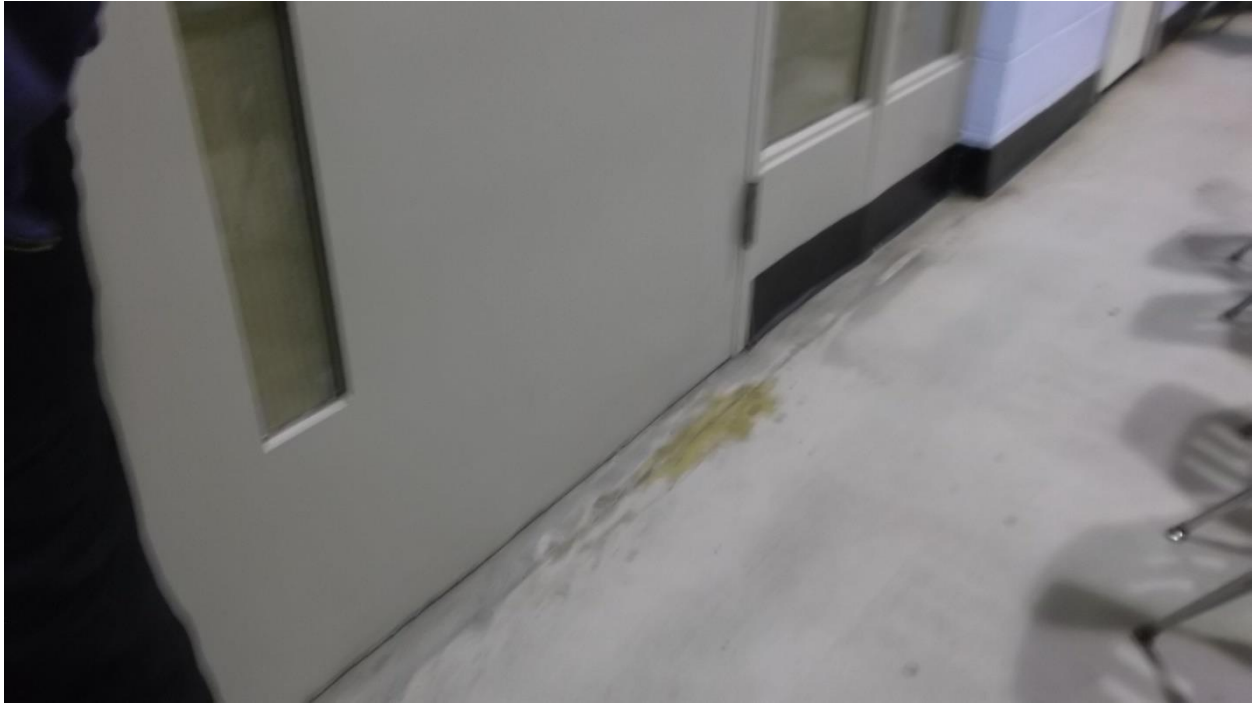
Gymnasium Worn Flooring along the Double Door Entrance Wall
