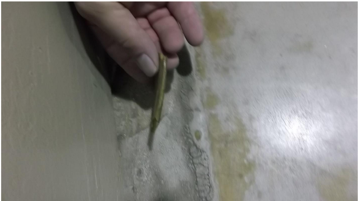
Gymnasium torn Flooring along the inside Wall
