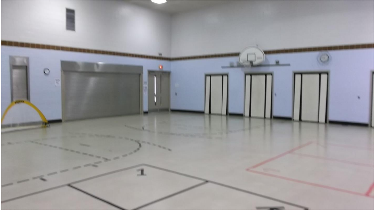
Gymnasium Rubber Floor to be replaced
