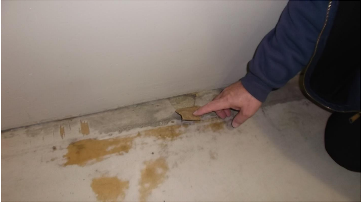
Gymnasium torn Flooring along the inside Wall
