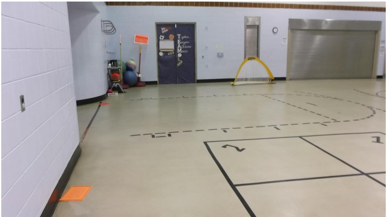
Gymnasium Rubber Floor to be replaced
