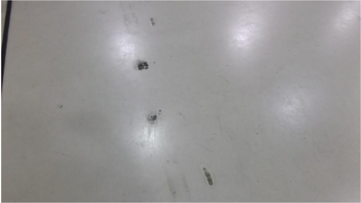
Gymnasium Worn Flooring under Basketball Hoop
