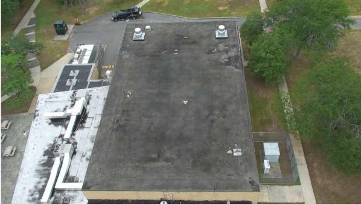
Existing Ivy Hall Roof - Existing Upper Flat Roof over the existing gymnasium.
