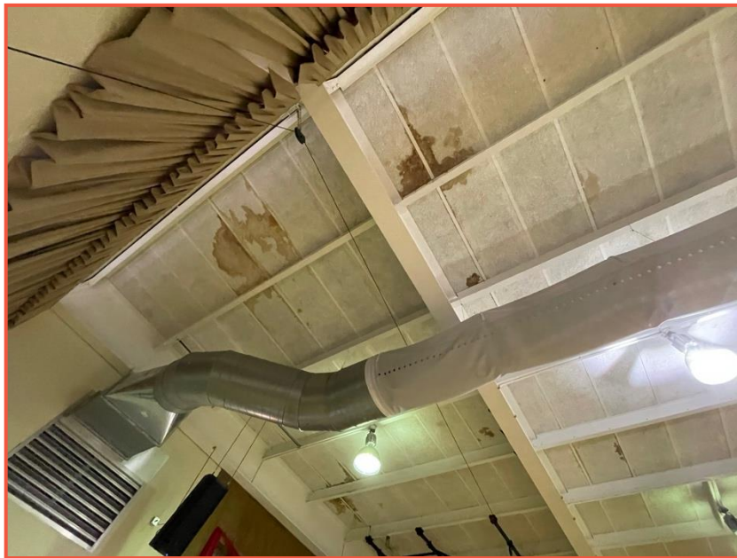
Photo No 6. Ivy Roof Underside – Typical staining
