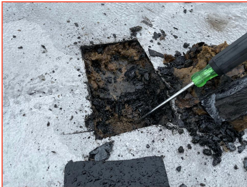
Photo No 2. Ancorage Roof Probe – Water under all 3 roof membranes
