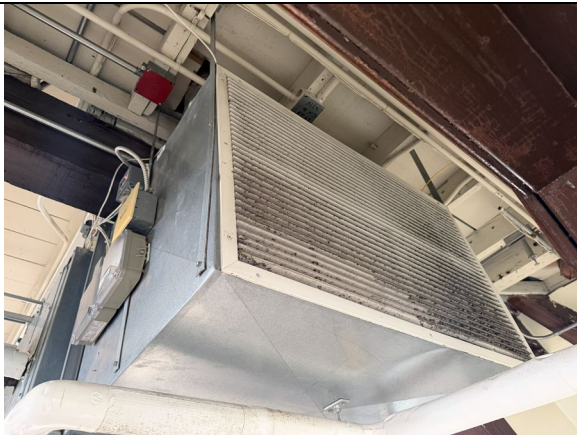
Picture 7: Typical FCU plenum return grill
