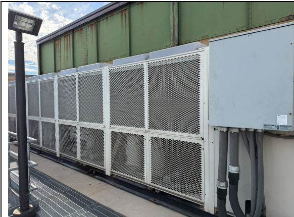
Picture 1: Air cooled chiller on elevated platform in exterior enclosure.
