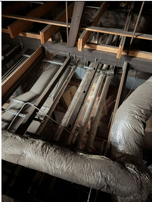
Picture 15: Missing or incorrectly installed insulation in the attic
