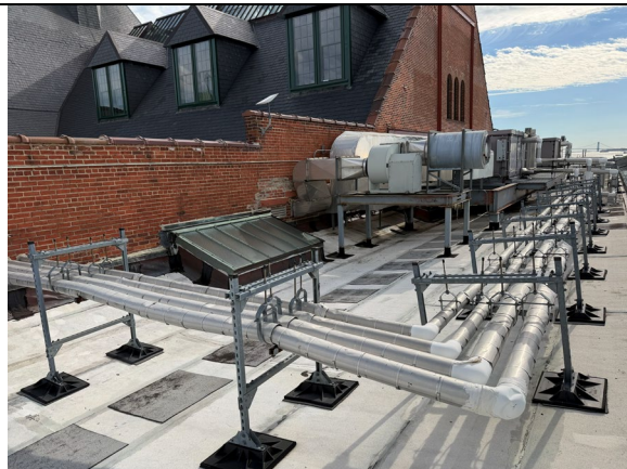
Picture 12: RTUs and EF on roof
