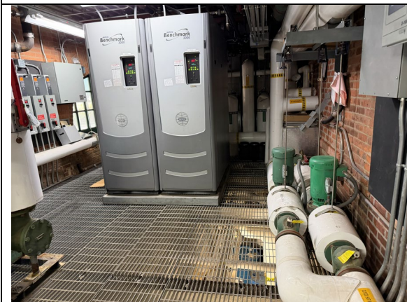
Picture 3: Existing boilers
