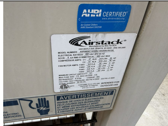
Picture 2: Air cooled chiller nameplate
