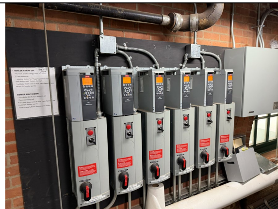
Picture 4: Existing boiler pump VFDs
