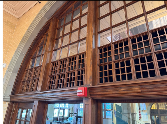
Picture 14: Typical wood slat grills for supply and return in the main hall space
