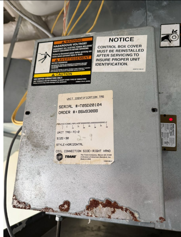
Picture 6: Typical FCU control panel
