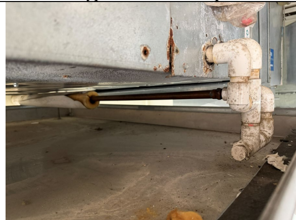
Picture 8: Condensate pipe without insulation below FCU
