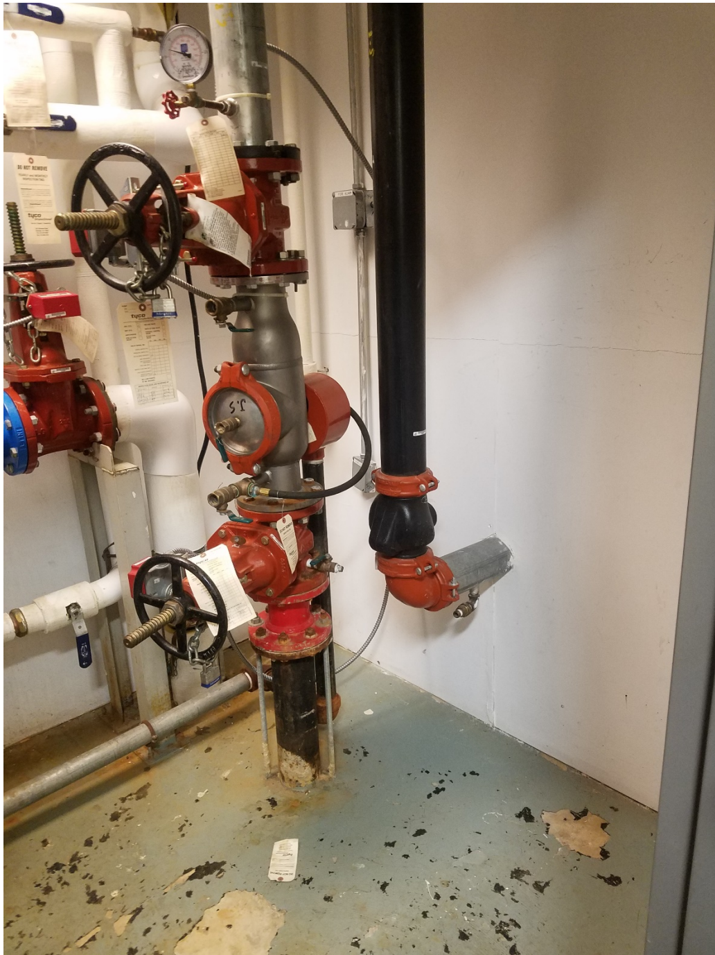
Existing Fire Water Entrance into the Building. EXHIBIT 'C'
