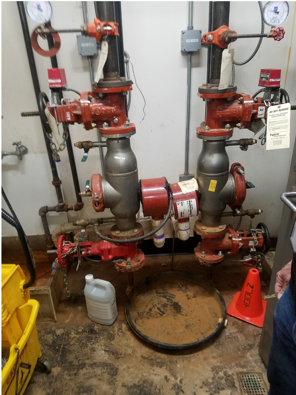
Sprinkler Equipment Room EXHIBIT 'C'
