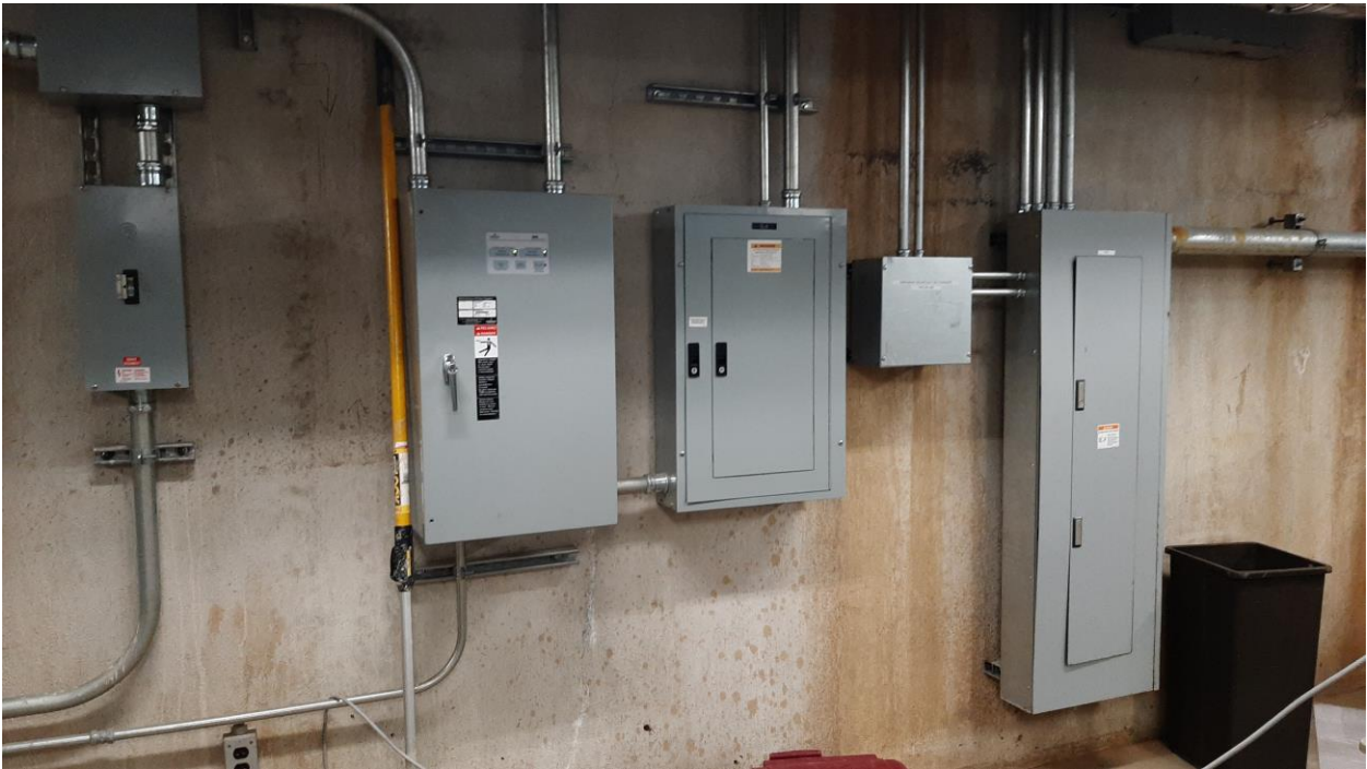
Existing Electrical Panels in Main Mechanical Room-Basement
