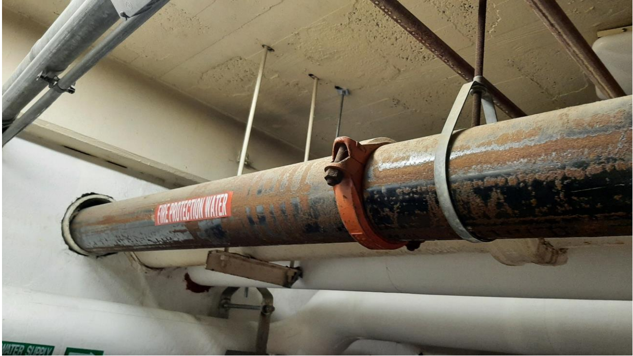
MOB Basement- Existing Fire Protection Water Pipe.
