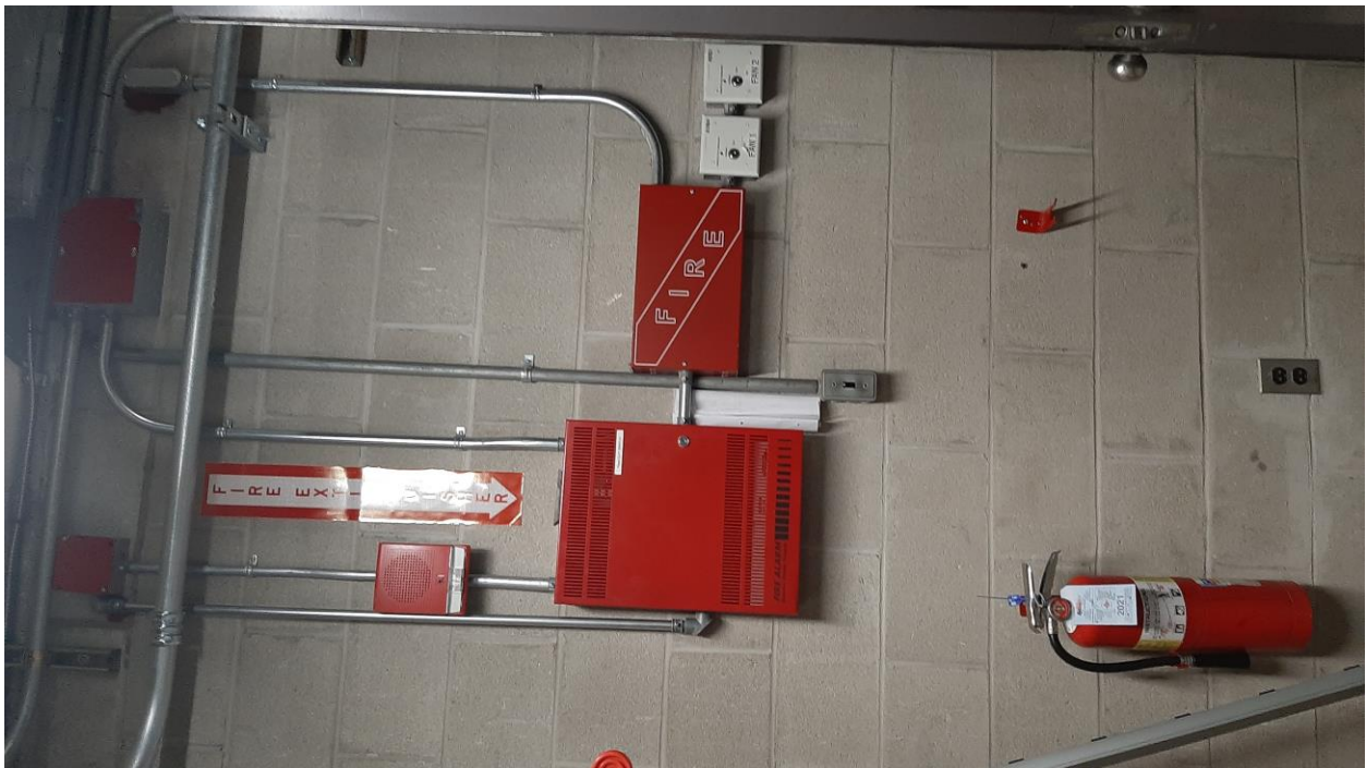
Existing Fire Alarm Panels at Third Floor-F&A Building.
