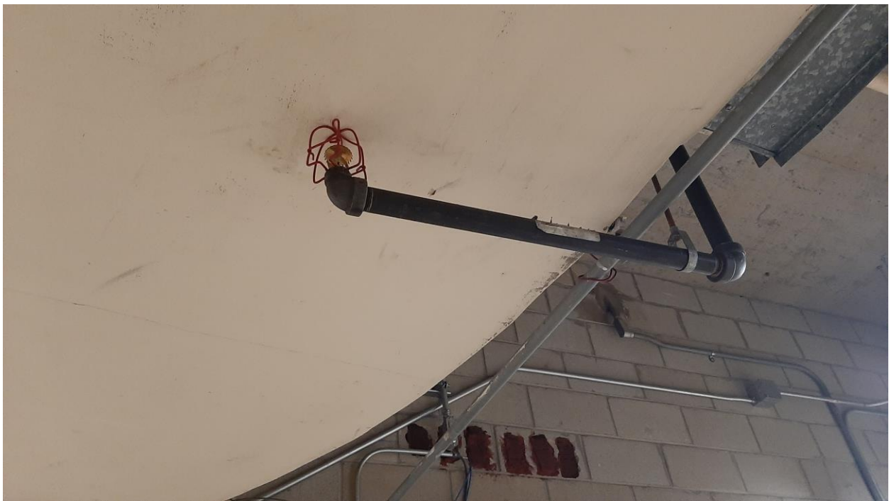
Existing Partial Sprinkler System Sprinkler Head- F&A Mechanical Room.
