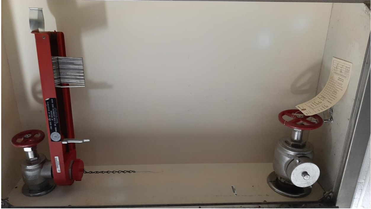
Existing Fire Department Valves at Third Floor.
