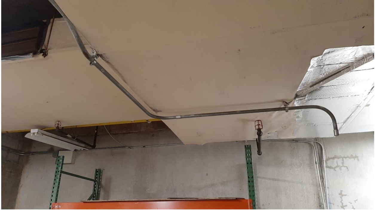
Existing Partial Sprinkler System Sprinkler Head- F&A Mechanical Room.
