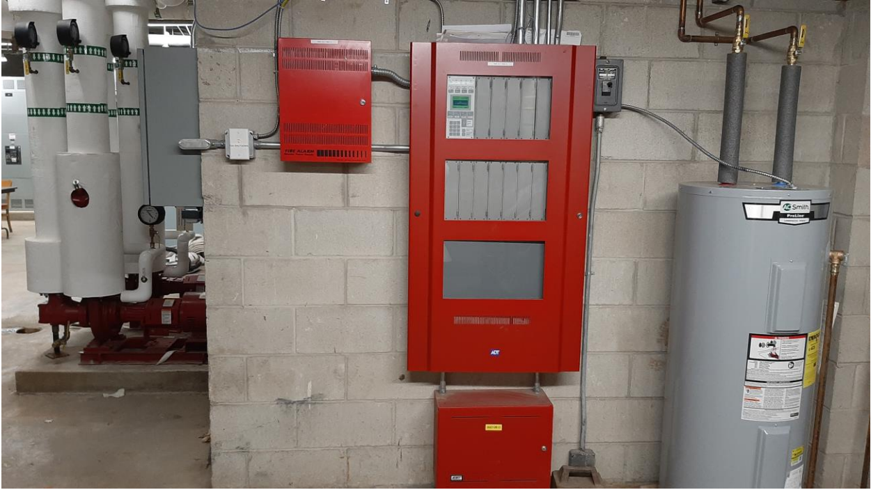
Existing Main Fire Alarm Panel in Basement in Main Mechanical Room.
