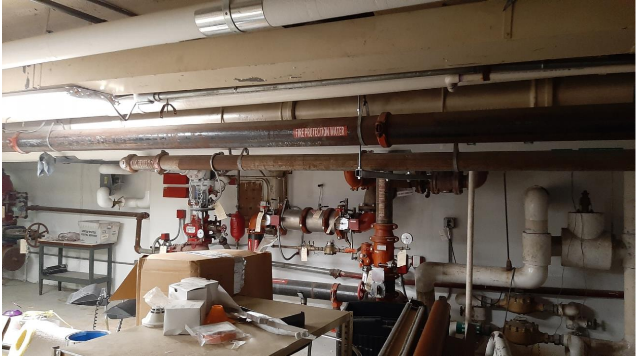
Main Office Building (MOB) Basement- Mechanical Room
