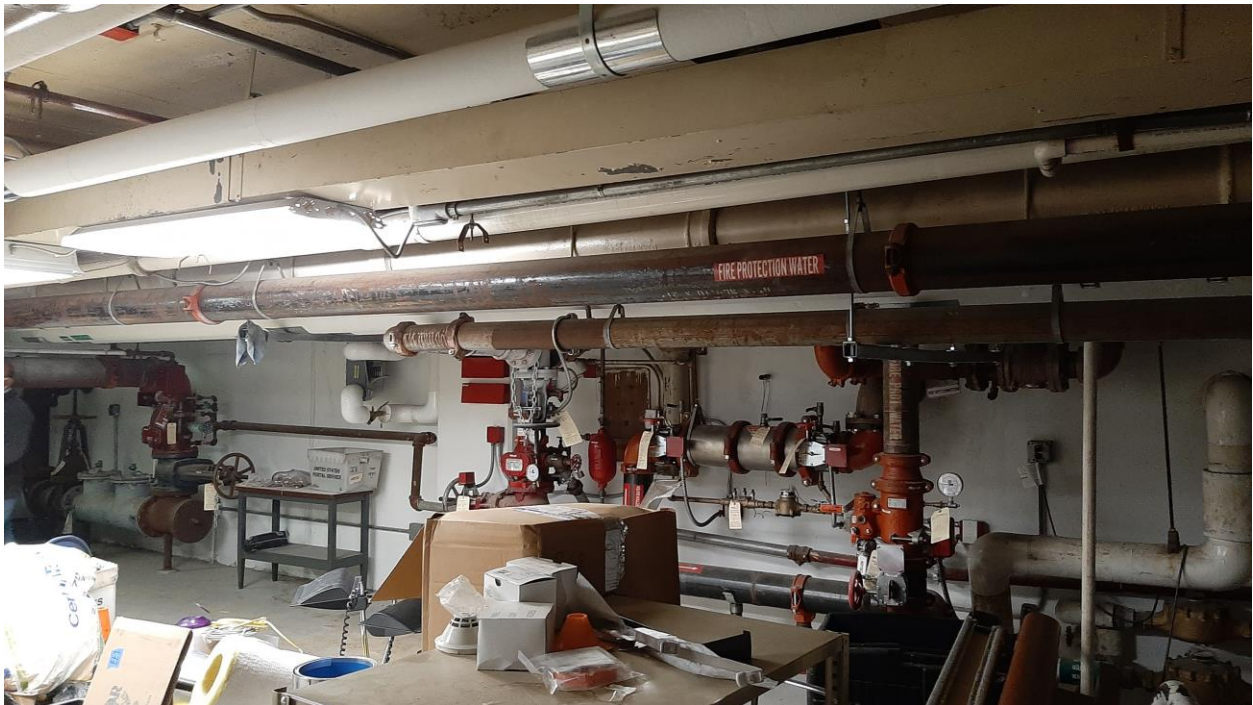
Main Office Building (MOB) Basement- Existing Partial Sprinkler System Water Main
