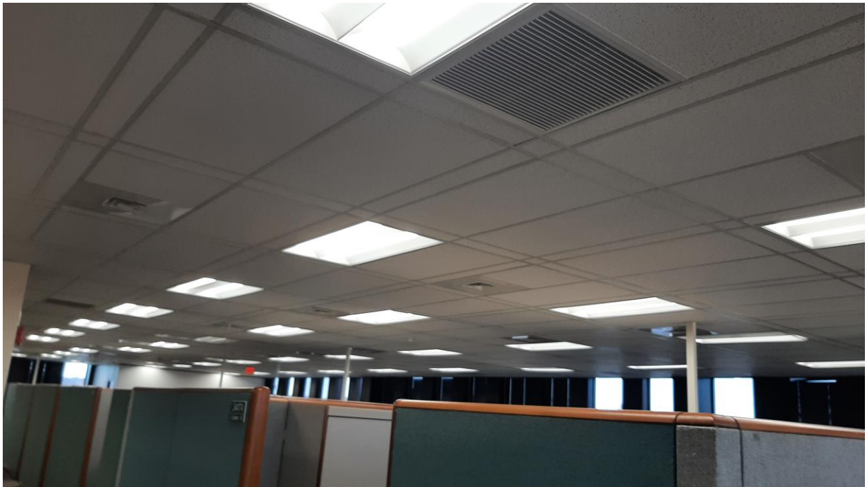
Existing Third Floor Suspended Ceiling System, Exit Signs, Lighting Fixtures and Diffusers.
