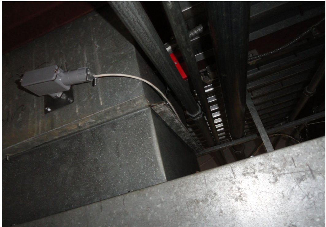
Outside air intake damper and sensor that need to be repaired for proper operation.
