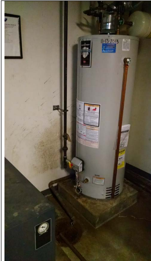
5. Mold Growing on Sheetrock wall In Mechanical Room
