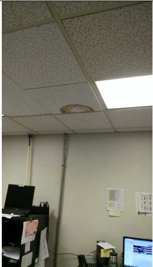
8. Water Stain on Ceiling Tile; Office Overseeing Lanes
