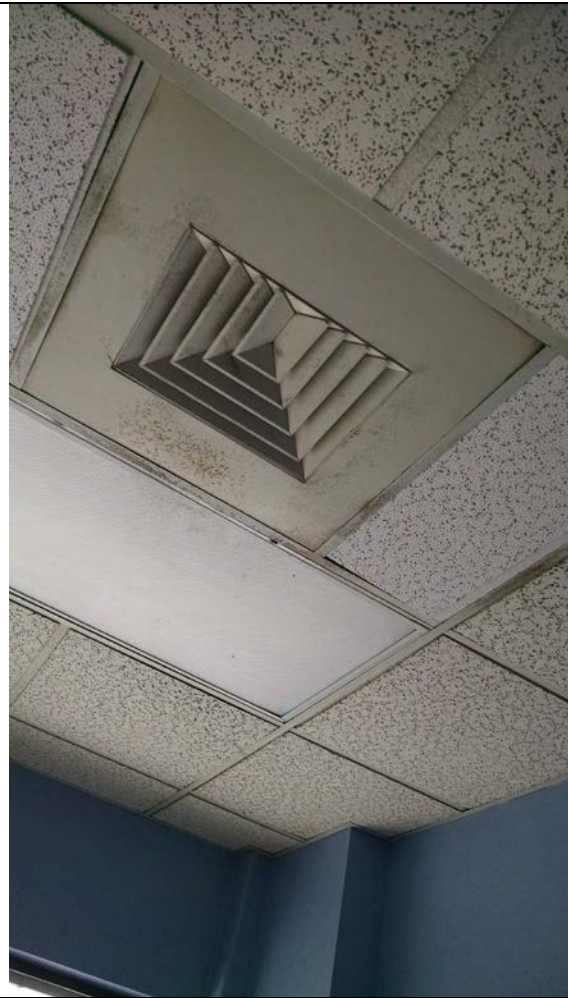
2. Mold Growing on Diffuser, Splines and Light Cover in Break Room
