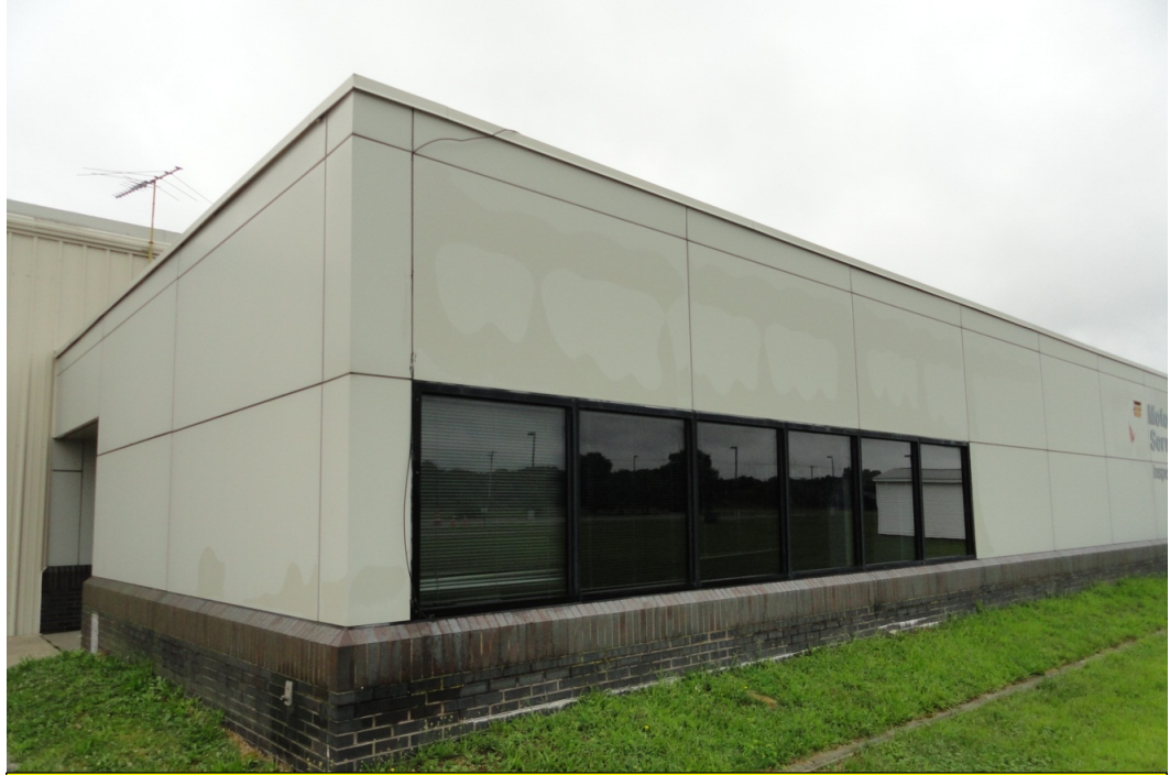
Outside of the building of break room. FRP panels are sweating due to the temperature inside of break room.
