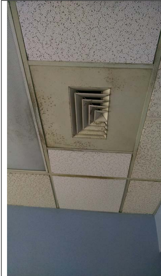
3. Mold Growing on Diffuser, Splines & Light Cover in Break Room
