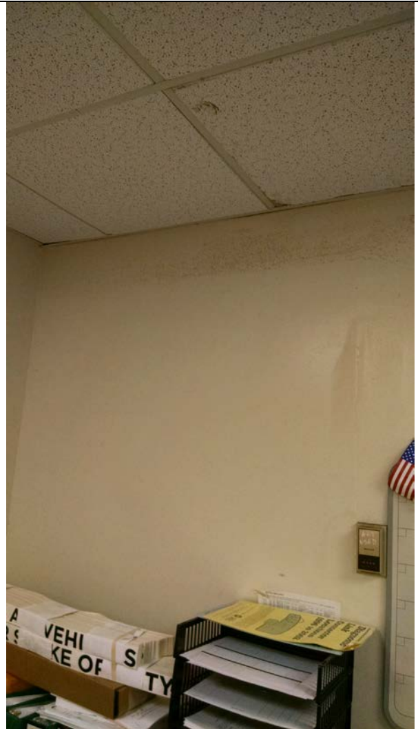
4. Mold Growing on Office Wall
