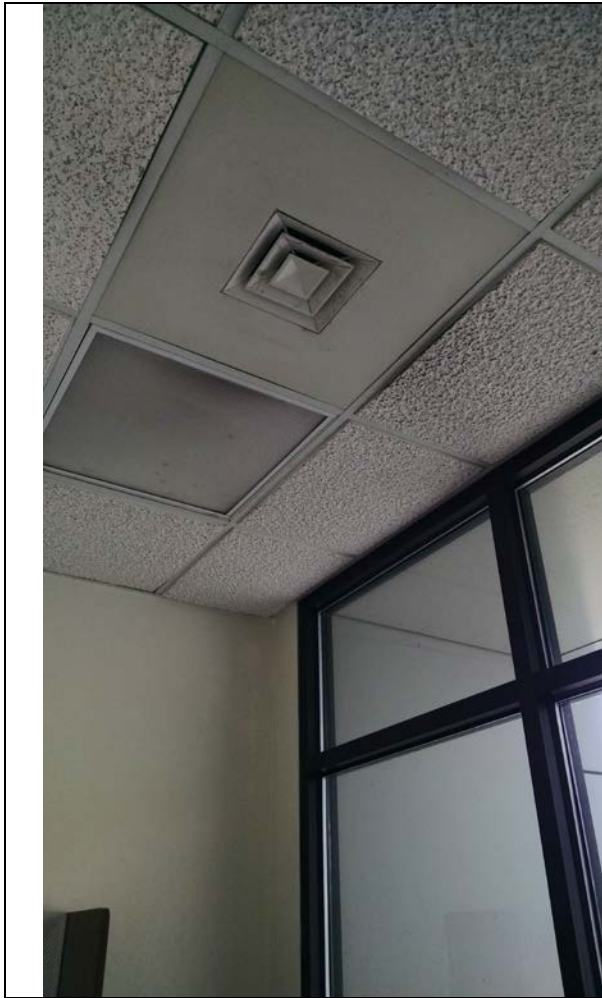
1. Mold Growing on Diffuser in Vestibule
