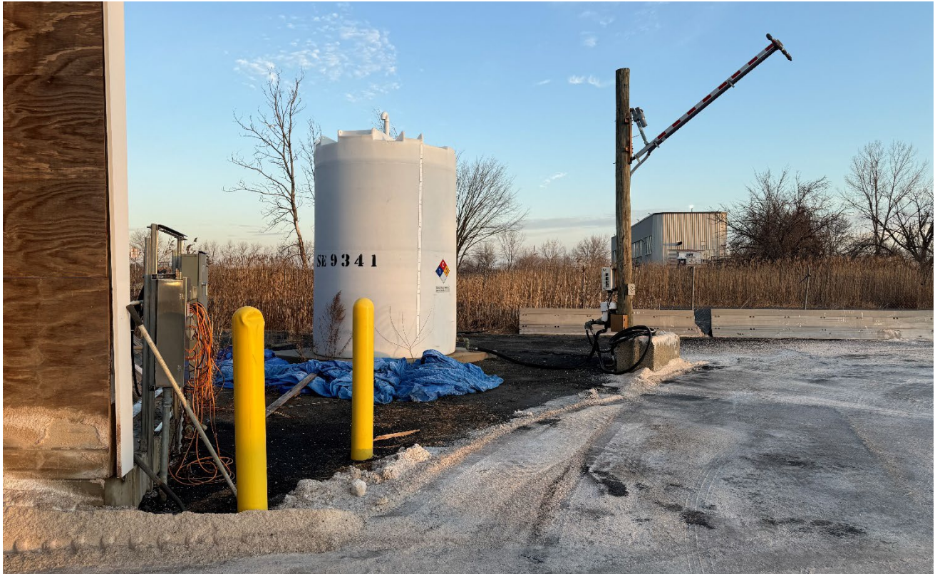
Existing Salt Wetting Arm and Calcium Tank
