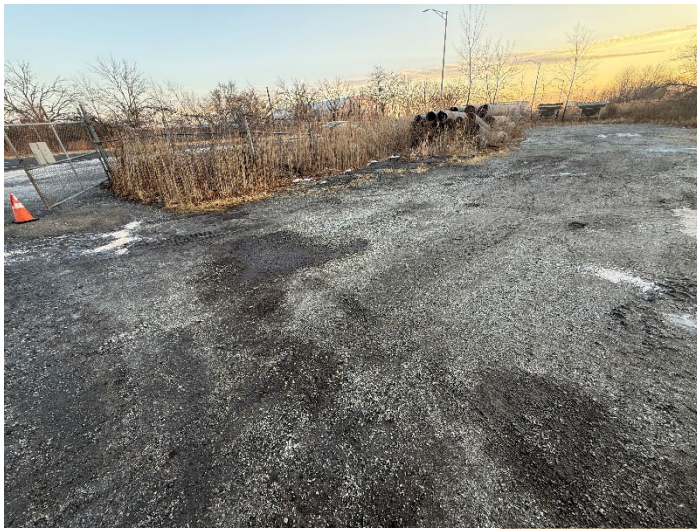
Left: Damaged Asphaltic Pavement
