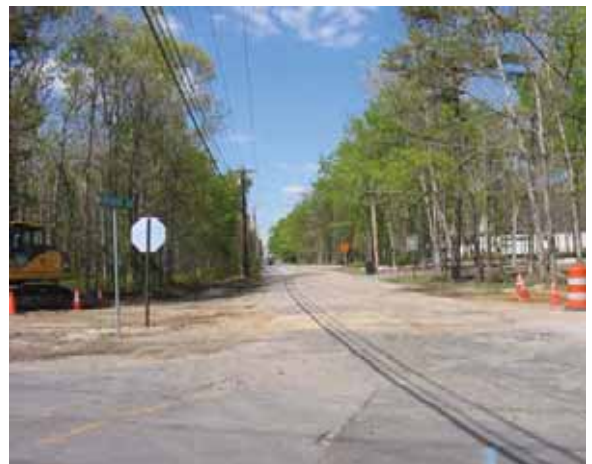
One of the many roads in the township that are being improved for new development.
